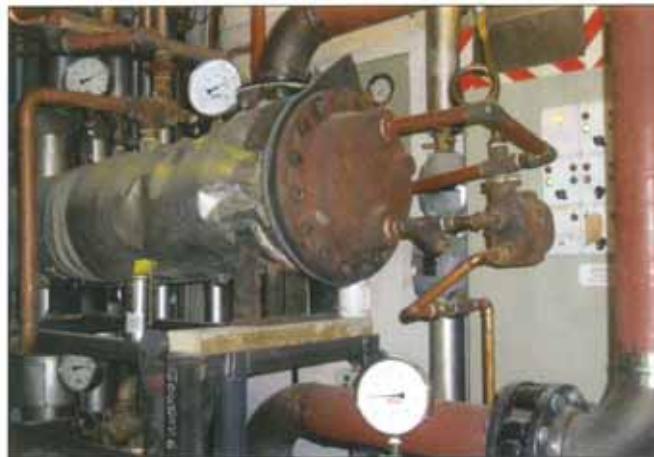
The old steam-powered heating calorifiers that have provided heating to the Women's Health & Maternity Unit.
