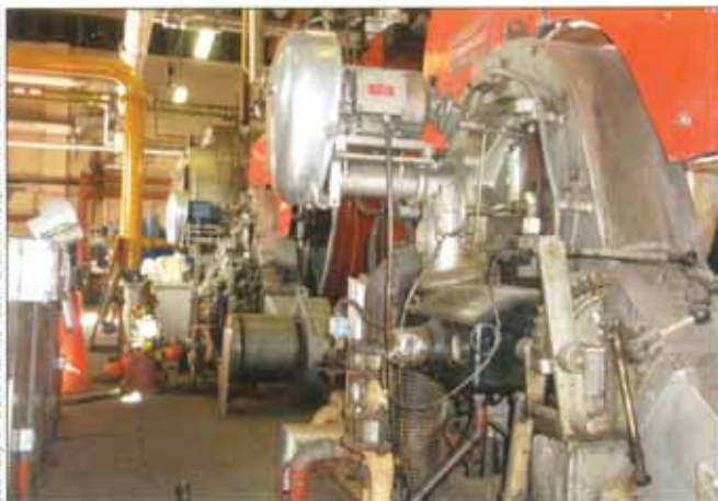
Existing steam boilers in the main boiler room – two Cradley Steampacket units installed in 1994, and an older Yorkshireman.
