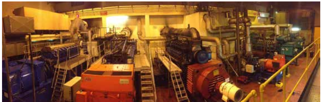
Museum of CHP: the impressive generating room houses an array of plant from the 1970s to more recent times
